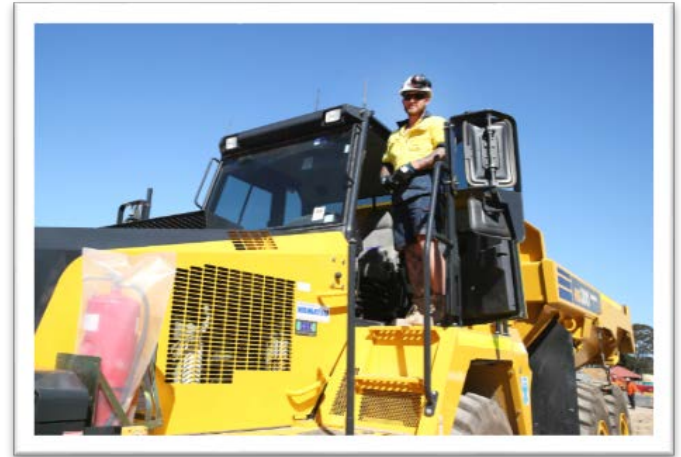
A tipper truck supports excavation for the Prince of Wales Acute Services Building
