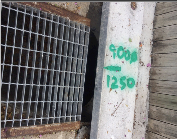
Figure 9. Storm water drain showing depth of trench and width of pipe at the end of Eurimbla Avenue
