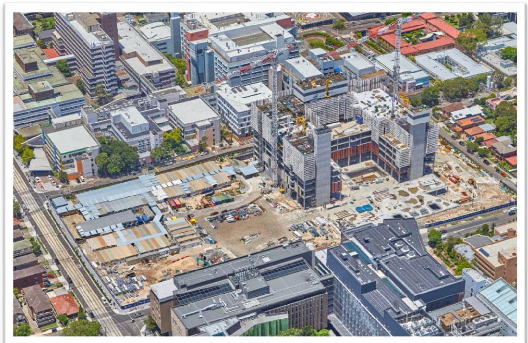
The Integrated Acute Services Building construction site viewed from Botany Street Randwick
